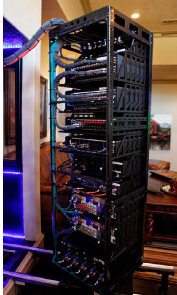
Visitors get hands-on experience using smart home systems, touchpanels, and iPad controls, and can check out live system hardware up close and personally.
